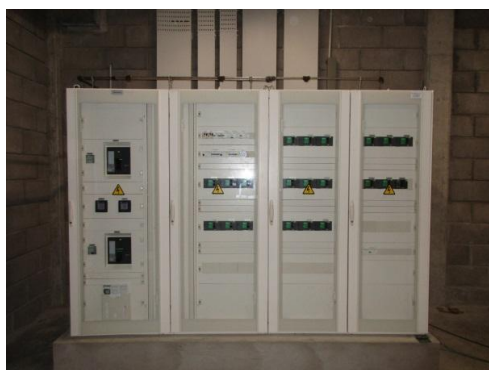
Illustration 13. Main distribution board
