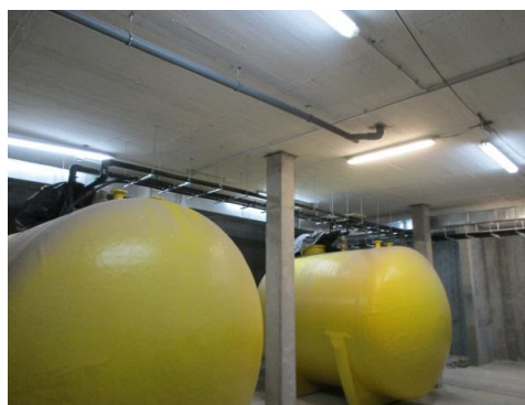
Illustration 14. Diesel oil tanks
