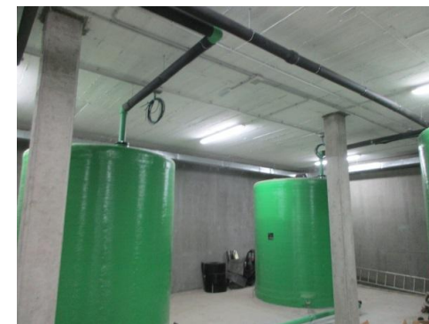
Illustration 12. Sea water tanks
