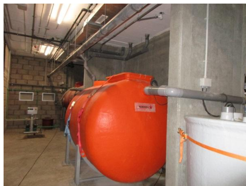
Illustration 10. Reverse osmosis plant
