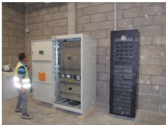
Figure 57. Power source module on the platform
